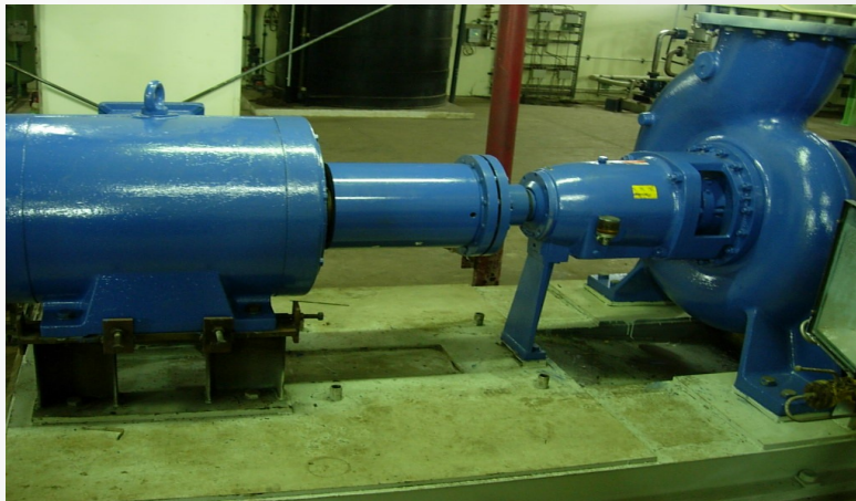
Secondary Cooling Pumps
