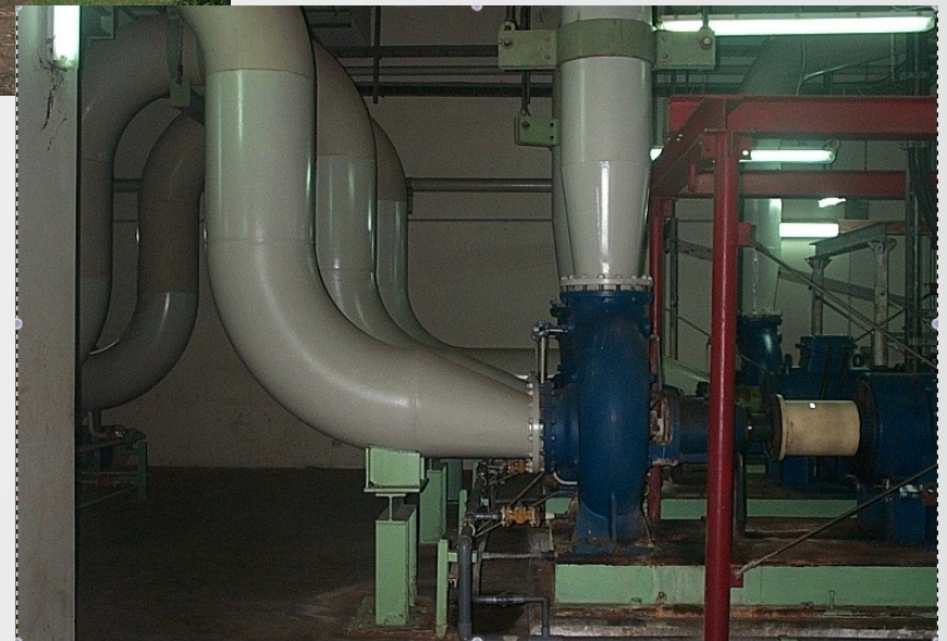
Secondary Piping System
